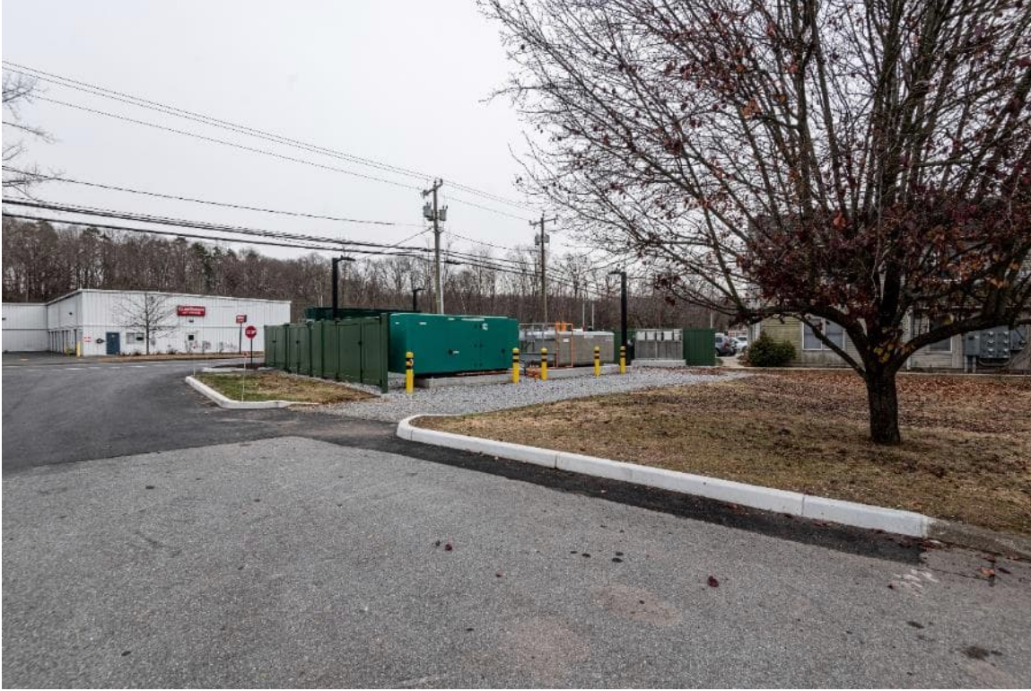
Pump Station Looking Southeast
