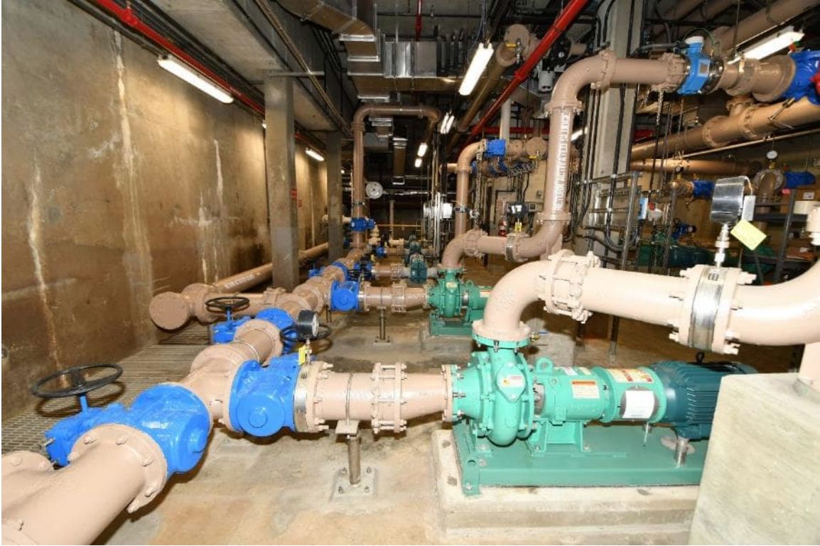
Operations Building Pump Gallery
