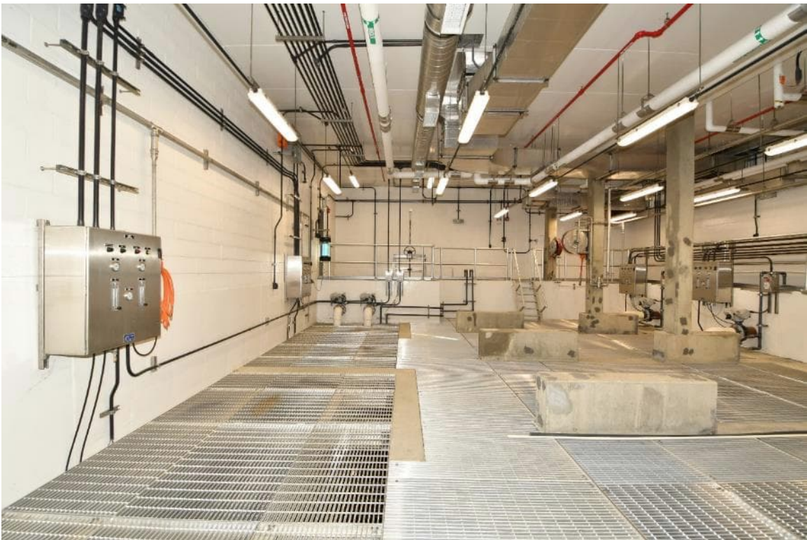
Operations Building Tertiary Phosphorus Removal Filter Room
