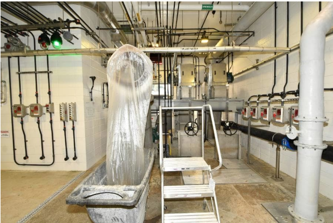
Influent Building Showing the Influent Screen and Washpress
