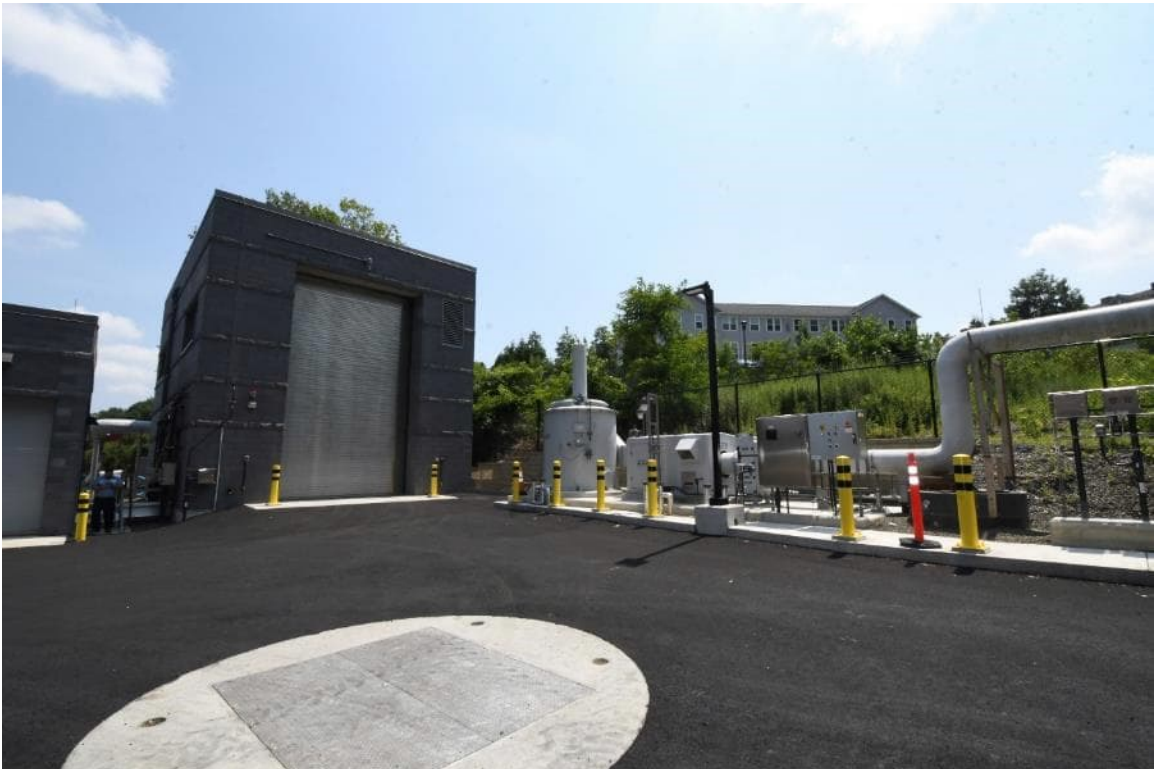
Septage Receiving Building and Odor Control No. 1
